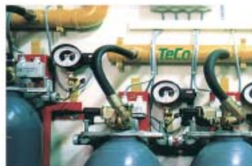
Total flooding FM-200 Extinguishing System Turn-key project executed by TeCo
