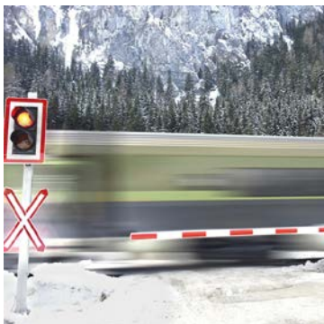
Level crossing safety system
