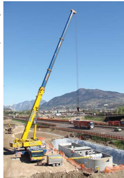
© SW Umwelttechnik, Water protection system
