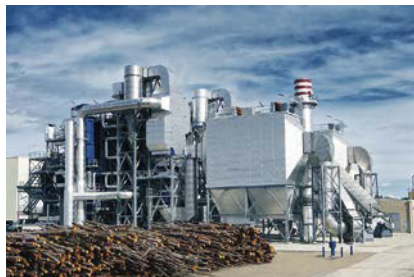
Flue gas cleaning, ESP/electrostatic precipitator
