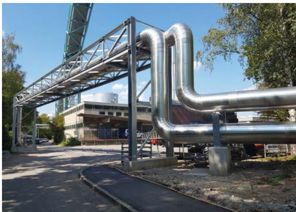
Turnkey solutions are core business © Bilfinger Industrial Services GmbH
