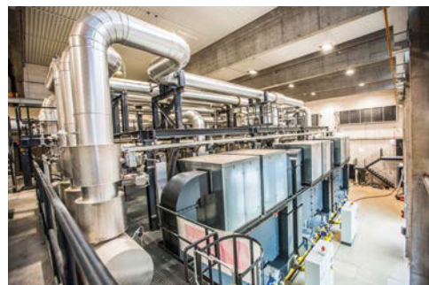
Heating plant Klagenfurt
